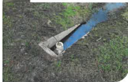
Pipe that had become obstructed.
